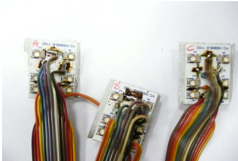
Figure 4. Cabling for Philips MASTERLEDs.
